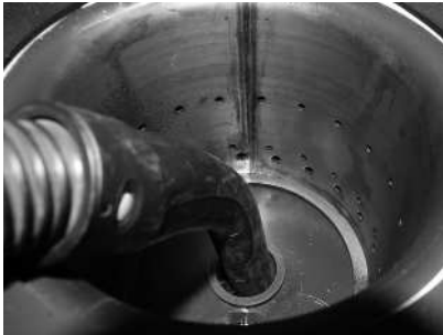
Fig. 48 Vacuum out the primary air tube in the centre of the burner bowl
